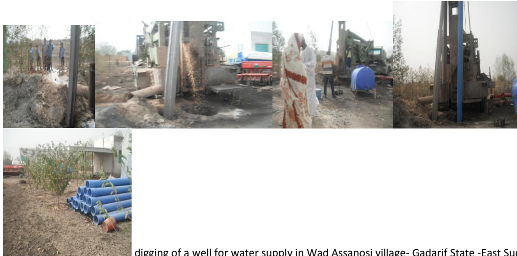
digging of a well for water supply in Wad Assanosi village- Gadarif State -East Sudan.
